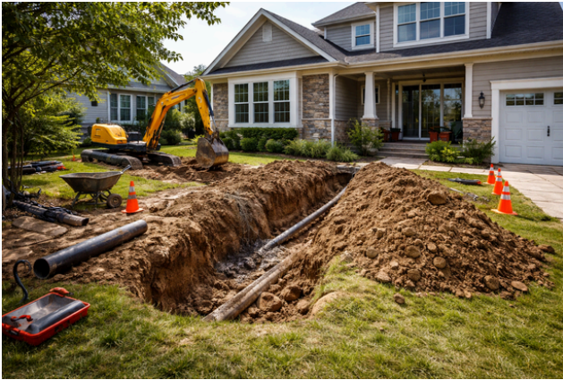
BEFORE (DIG - DAMAGED YARD)
