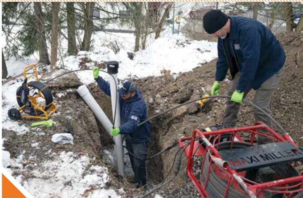
▲ Shelton Plumbing technician Frank Roberts, left, uses a Hathorn camera reel while company owner Josh Shelton uses a Picote Maxi Miller drain cleaning machine as they prep a sewer line for trenchless lining installation.
